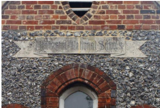
Pictures 16-17. Bennington School Parts of the building are visually most worthy of retention. Note spelling of Bennington (with double n) in centrally located stone detail.
