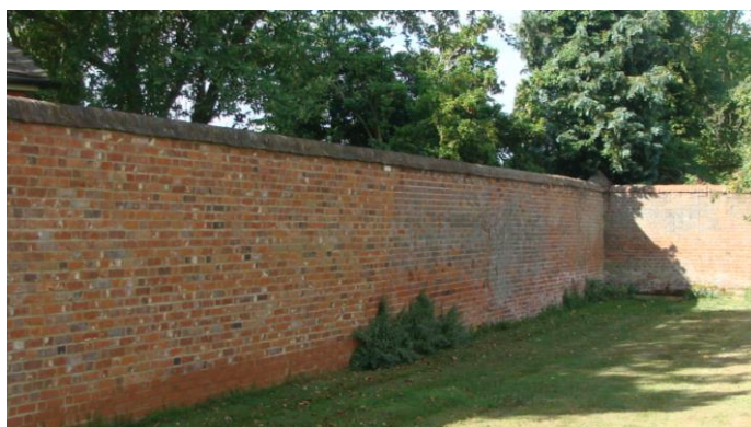
Pictures 31-33. Former kitchen garden at Bury Lodge Farm. Top traditional box edgings which the owners are encouraged to retain. Below walls about 3m in height, some repairs desirable. Grant assistance may be available.
